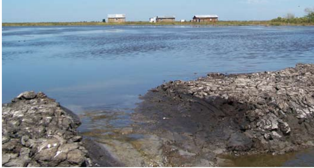
As sediment settles, water flows out of the project area through gaps in the containment dikes. Because particles settle at different rates, a small amount of sediment flows out with the water and is lost during the dewatering process. Engineers take this sediment loss into account when they calculate the amount of slurry they must pump to achieve target elevation.
