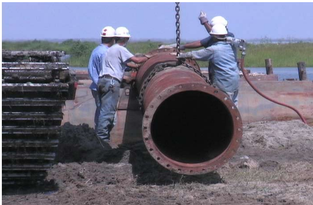
Workers connect 20-foot sections of pipe to build a pipeline — typically two to five miles long — from borrow area to fill site.
