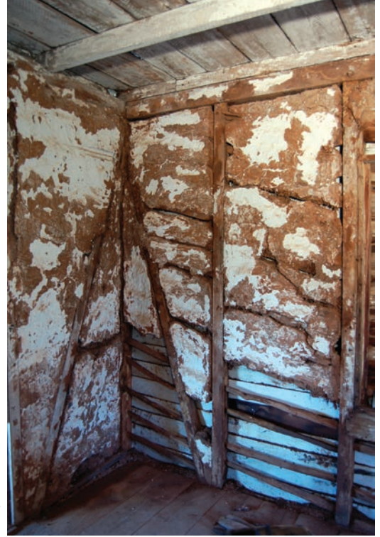
Bousillage, a mixture of mud and Spanish moss, was packed between timber frames and held in place with sticks to form walls of buildings. The dense material provided an insulating mass that moderated interior temperatures in both summer and winter.
