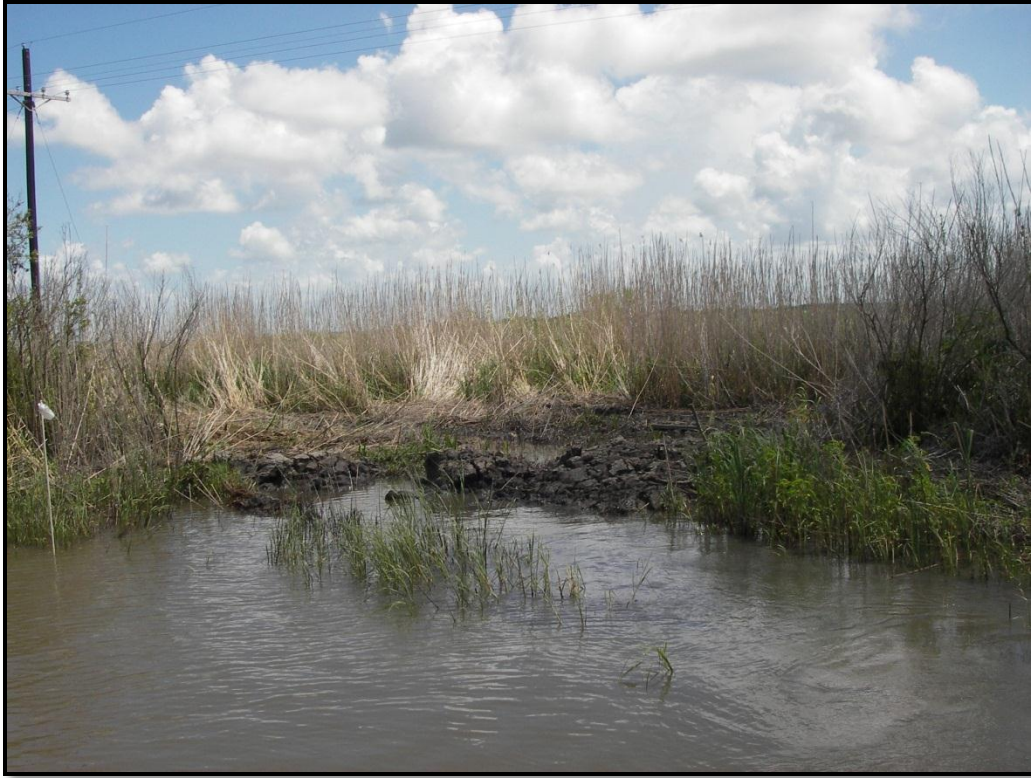
Photo No. 11, Damage to levee on Oaks Canal
