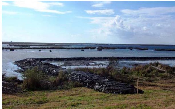
A view of the marsh creation project. The picture is taken from on top the hurricane protection levee at Galliano looking eastward over the broken marsh. The new levee marks the edge of the area being infilled by dredged sediments, which can be seen starting to fill the area.
