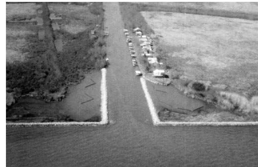
In addition to high-altitude aerial photography, DNR also obtains low-altitude images. This shot shows the Boston Canal-Vermilion Bay Shoreline Stabilization Project after the installation of rock breakwaters along Boston Canal. (DNR photo)
