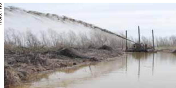
Spraying dredged sediment to restore marshes to specific elevations is one of the techniques used to reverse coastal wetland loss.
