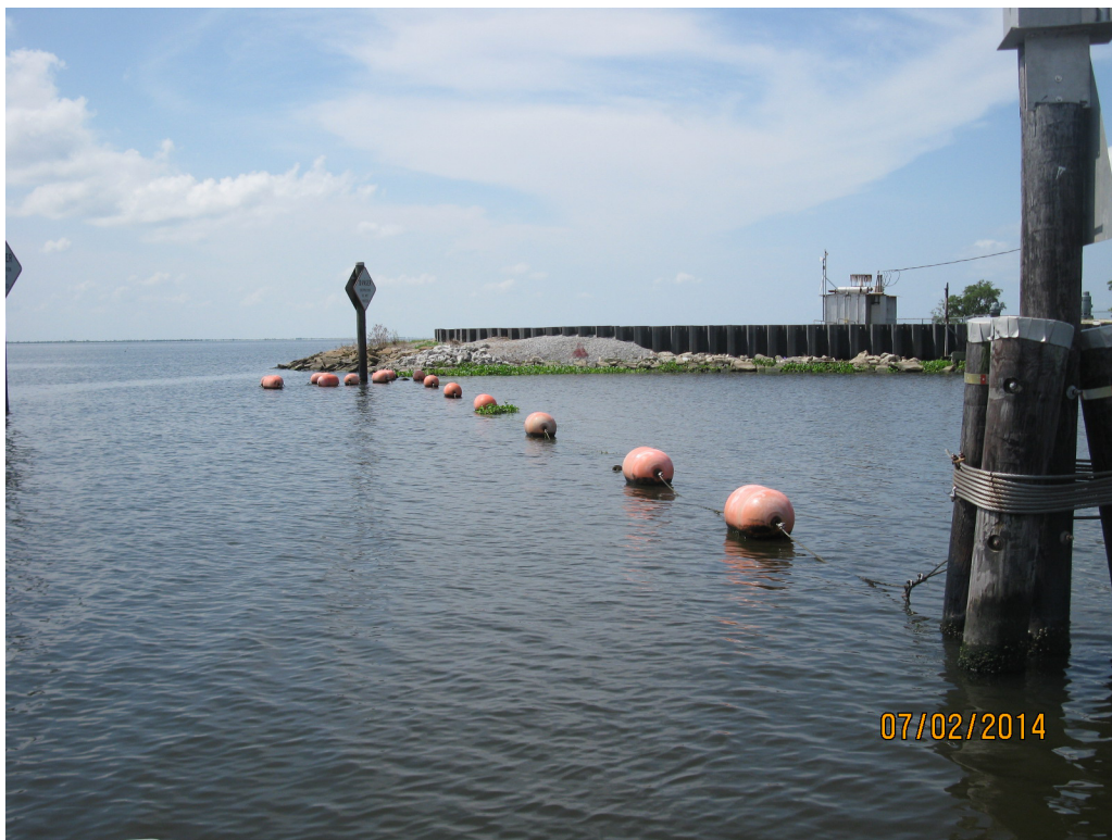
Photo #4 – Buoy Damage at Goose Bayou (South Side)
