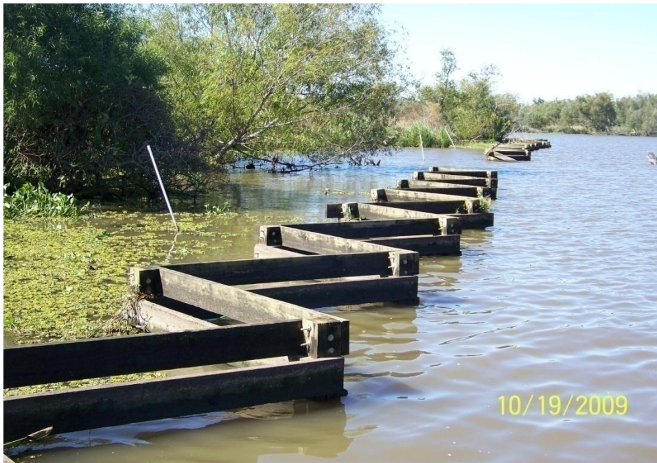
Photo No.34 – Site F2 - view of damaged fence units where a boat collided with the structure.
