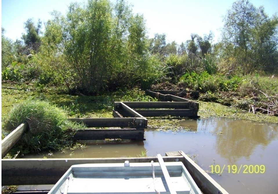
Photo No.39 – Site F1 – close-up of timber fence unit tie-in to bank on west side of structure.
