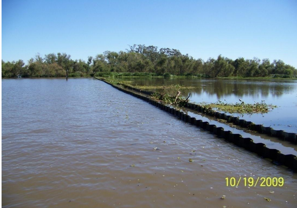
Photo No.61 – Site V1 – view along fiberglass sheet pile double wall looking eastward.
