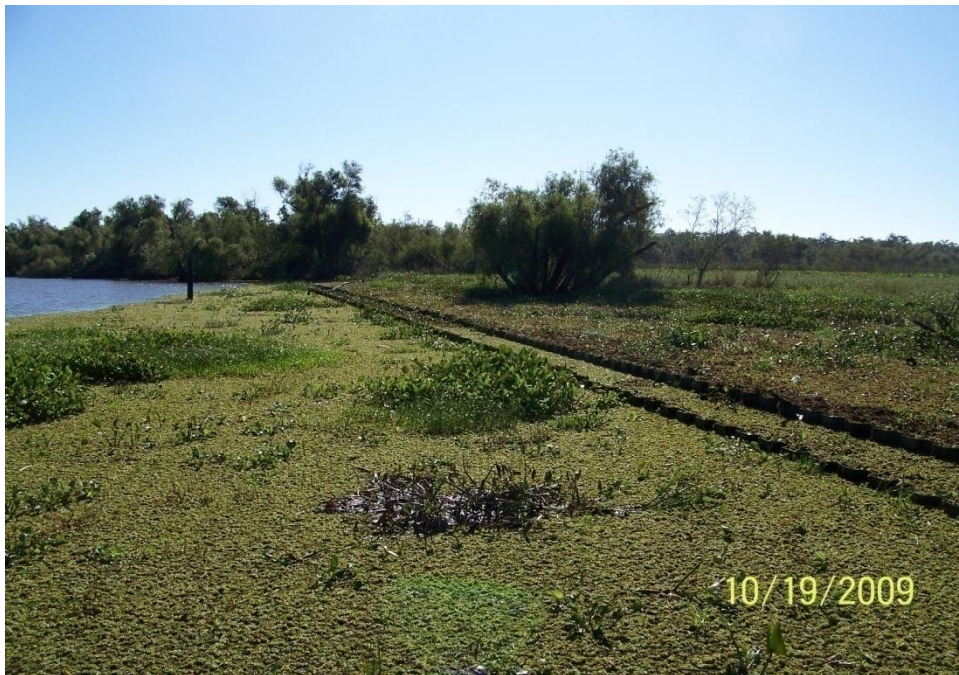
Photo No.14 – Site V2 - fiberglass sheet pile wall along south bank of GIWW looking east.
