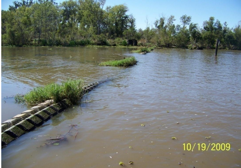
Photo No. 69- Site R1 – Areas that settled along Elevated Revetment Mats and CPE pipes.
