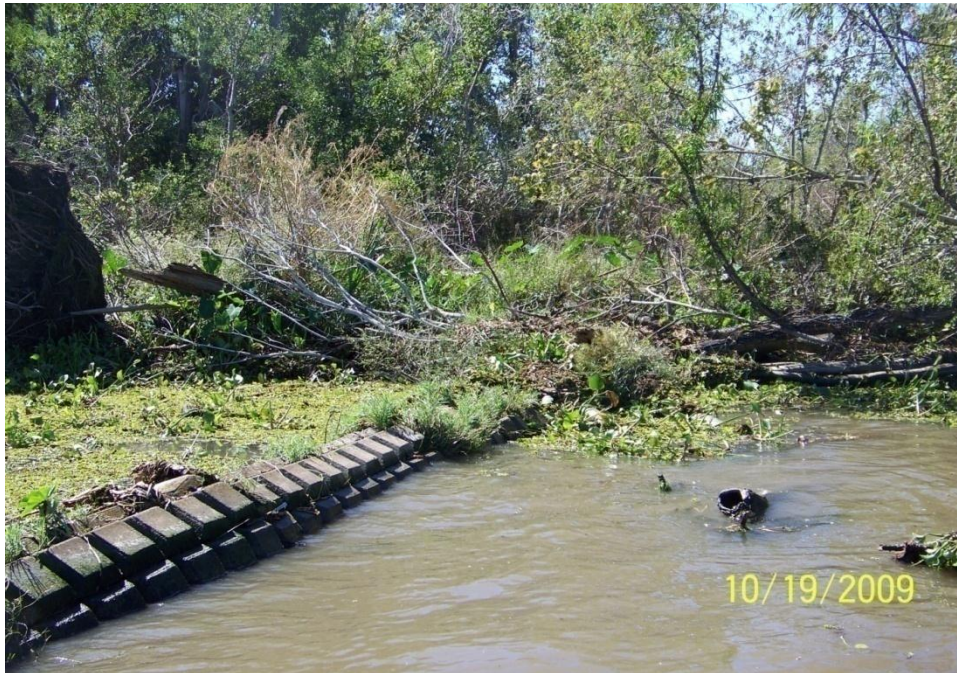
Photo No.66 – Site R1 – elevated shoreline system tie-in to bank on west side of structure.
