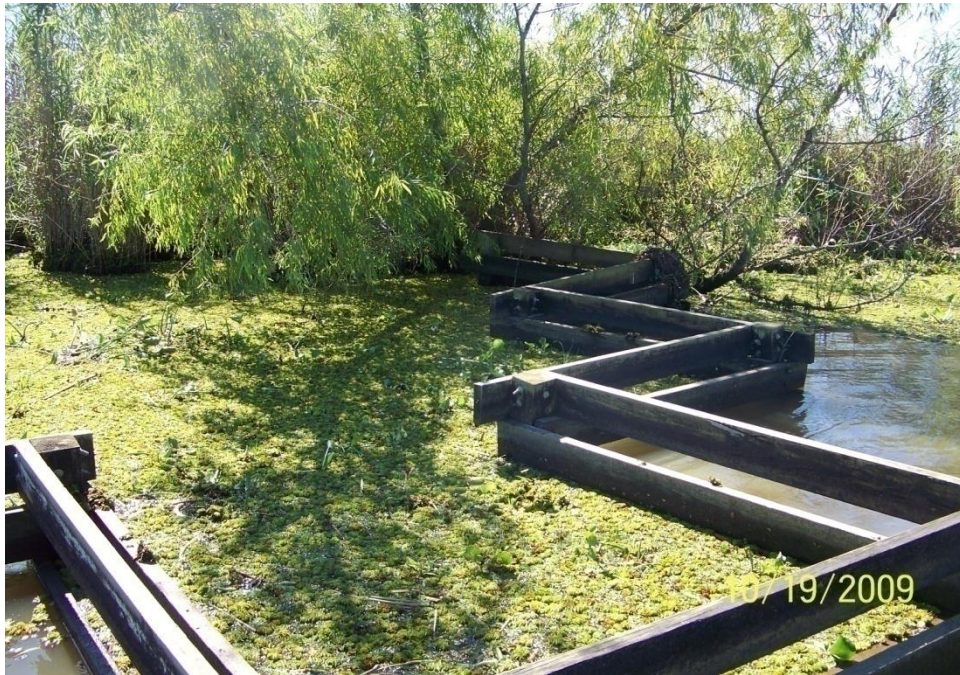
Photo No.36 – Site F1 – timber fence tie-in to bank on the west end of the structure.
