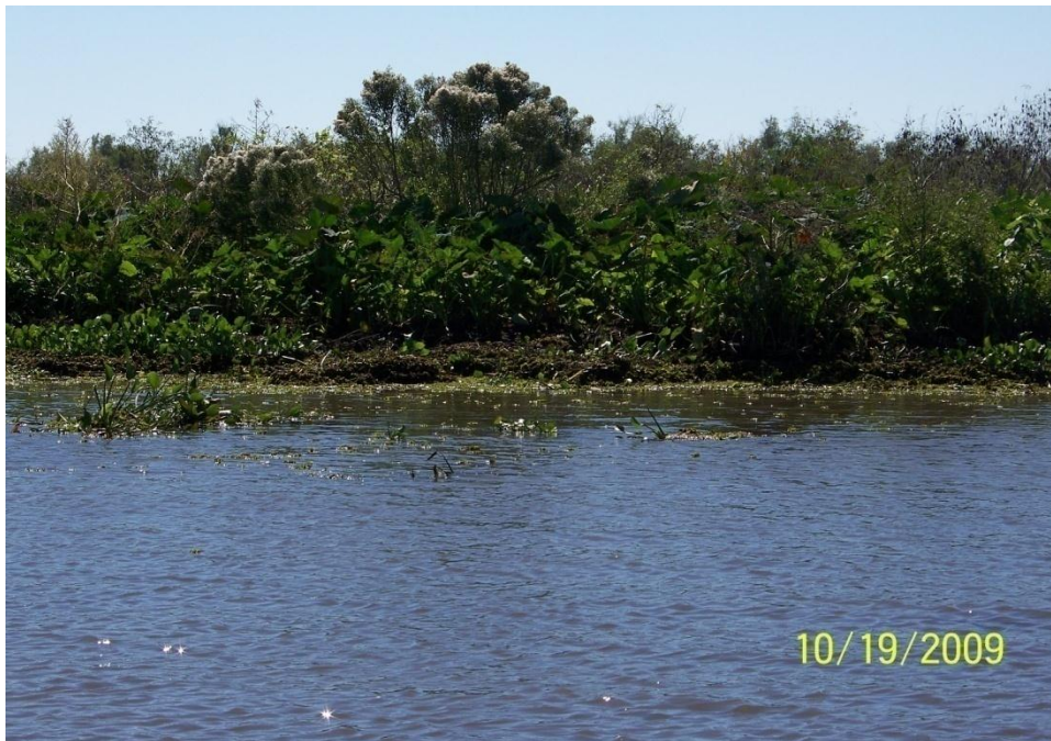
Photo No. 46 – Site J1 – view of accretion in front of double row concrete armor units.
