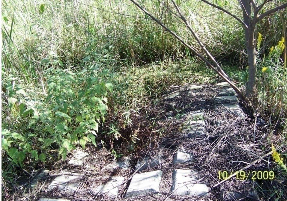
Photo No. 25 – Site A2 – armored earthen plug tie-in to bank on the east side of the structure.
