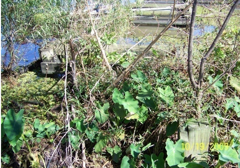
Photo No.29 – Site F2 – timber fence and vegetation growth on the west end of the structure.
