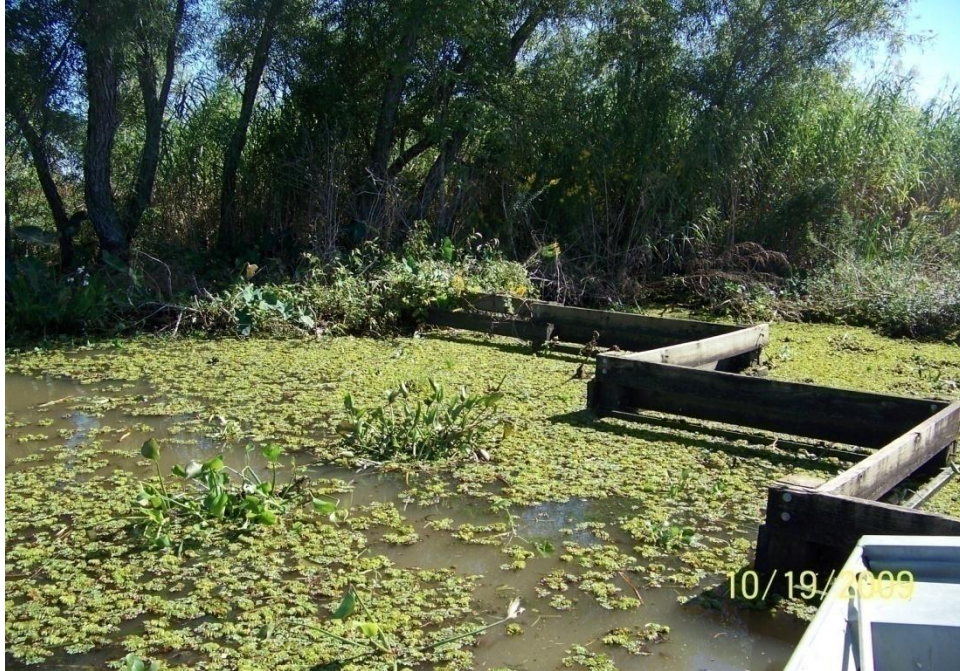
Photo No.35 – Site F2 – timber fence unit tie-in to bank on the west end of structure.
