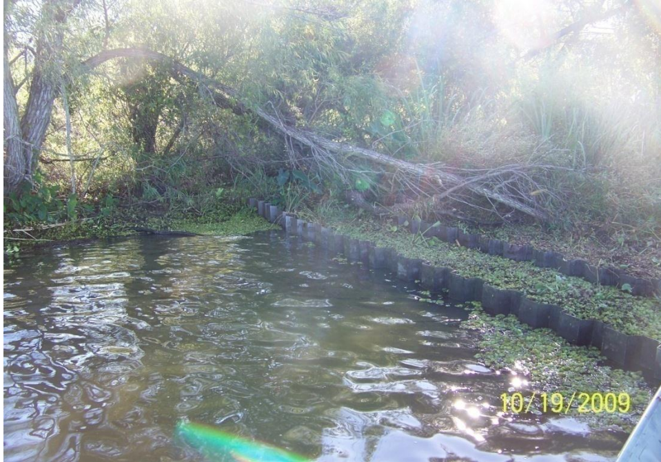
Photo No.5 - Site V3 – bank tie-in at the east end of the fiberglass sheet pile (double) wall.
