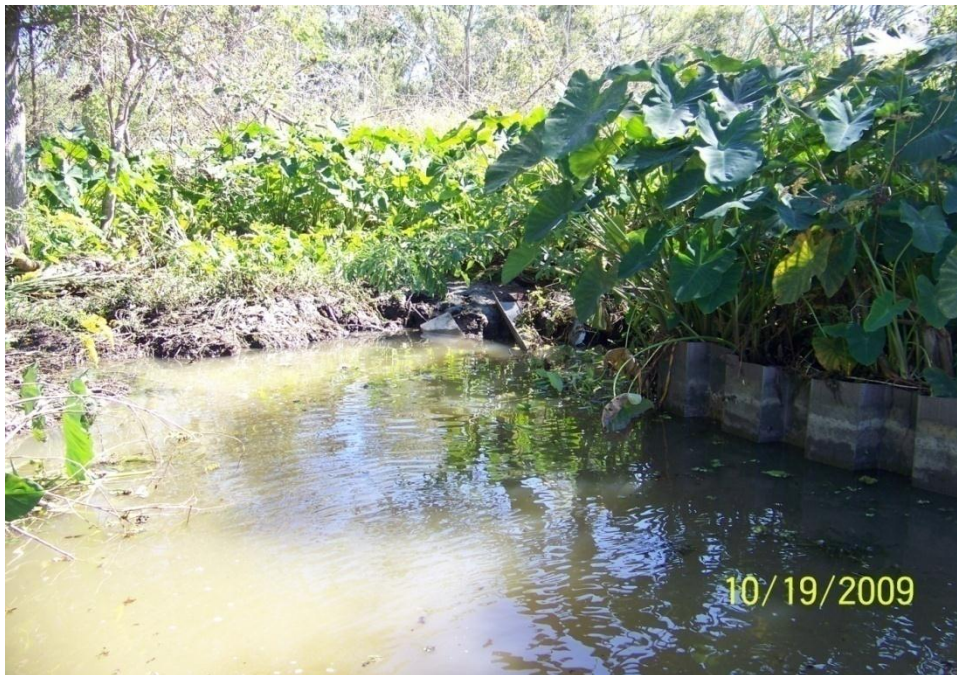
Photo No. 64 – Site V1 – fiberglass sheet pile double wall tie-in to bank on east side of structure.
