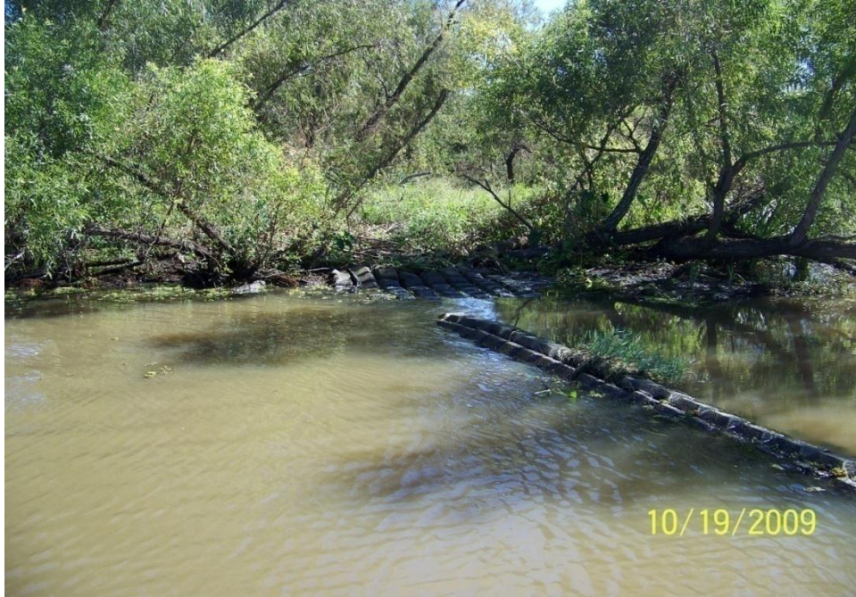
Photo No.57 – Site R2 – Elevation shoreline system (revetment & CPE) tie –in on the east side.
