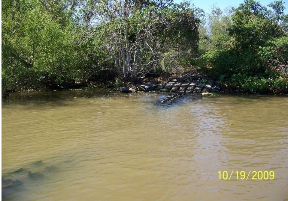
Photo No. 55 – Site R2 – Elevated shoreline system to bank tie-in on the west side of structure.
