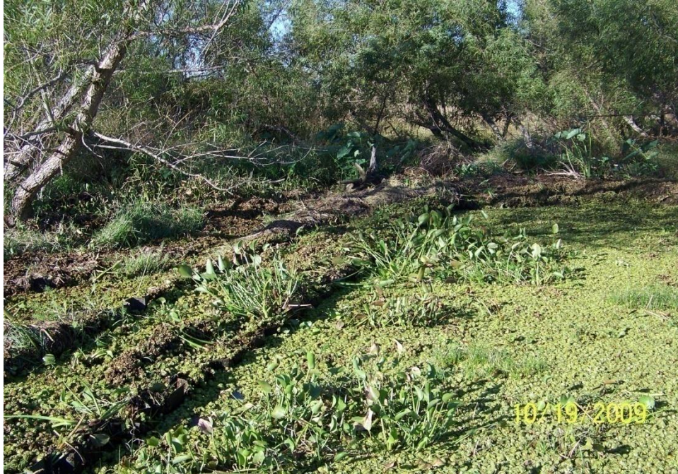
Photo No.3 – Site V3 – bank tie-in at the west end of the fiberglass sheet pile (double) wall.
