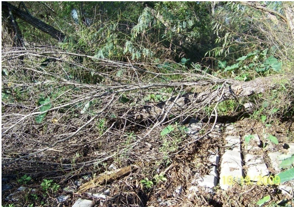
Photo No. 8 – Site A3 – close-up of the articulated concrete mats covering the earthen plug.
