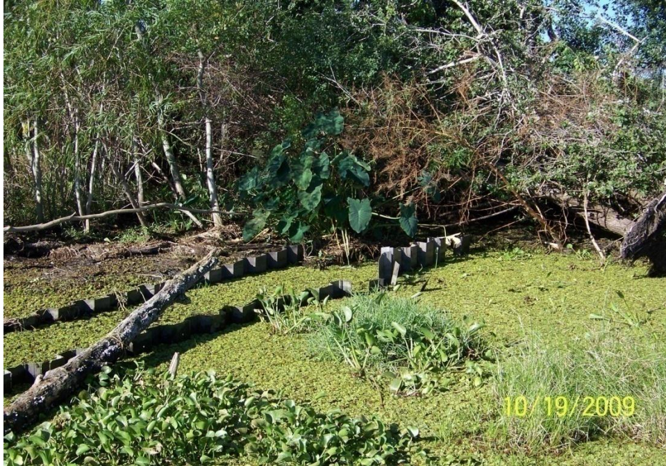
Photo No.13 – Site V2 – fiberglass sheet pile tie-in to bank on the west side of the structure.
