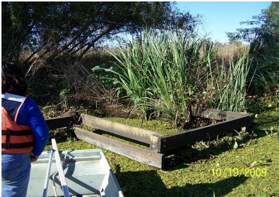
Photo No.18 – Site F3 – timber fence tie-in the bank line on the west side of the structure.
