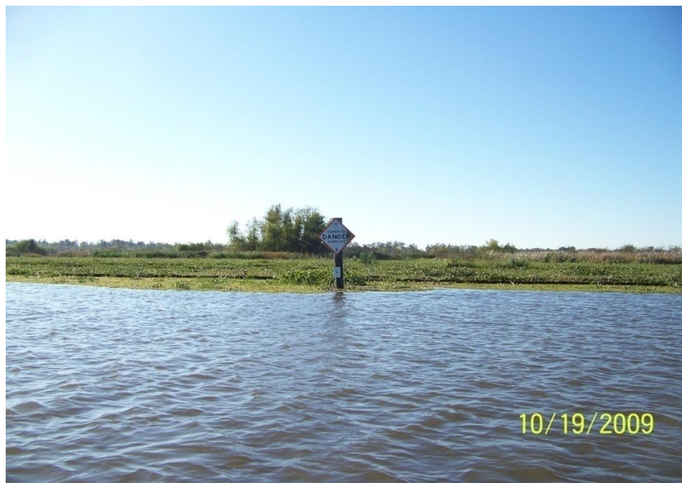
Photo No.2 - Site V3 – warning sign in front of fiberglass sheet pile (double) wall structure.
