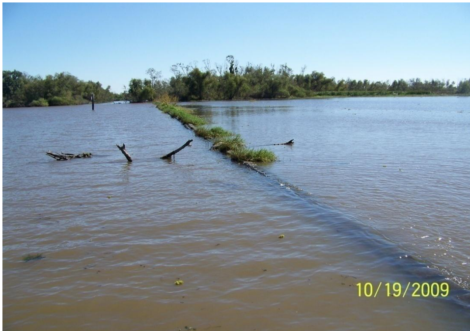
Photo No.50 – Site R1 – view of submerged revetment mats and CPE pipe looking east.
