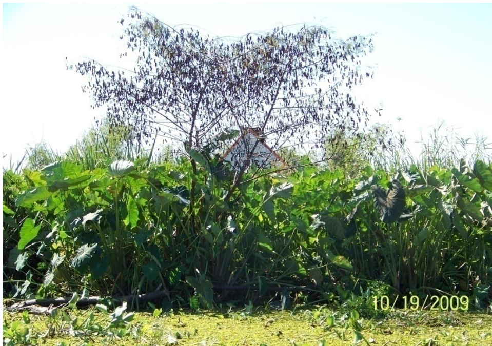
Photo No. 44 - Site J2 – view of warning sign and vegetative accretion in front of armoring units.
