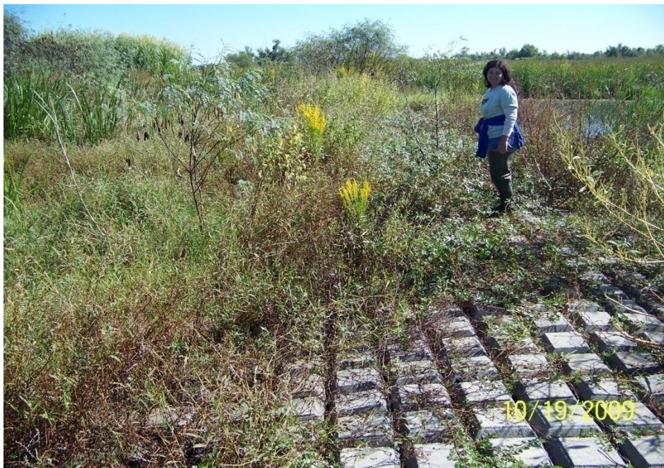
Photo No.24 – Site A2 – view of vegetative growth through the armored earthen plug structure.
