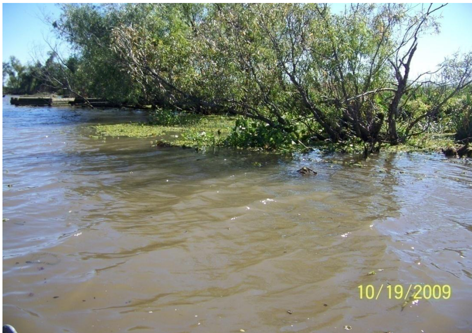
Photo No.32 – Site J3 – view of submerged double row concrete armoring units.
