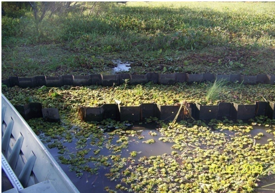
Photo No.6 – Site V3 – close-up view of fiberglass sheet pile (double) wall structure.
