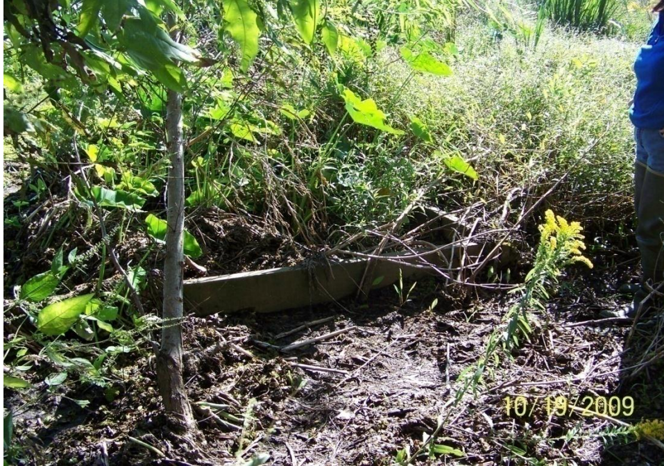
Photo No.21 – Site F3 – accretion in front and up to the top of the timber fence structure.
