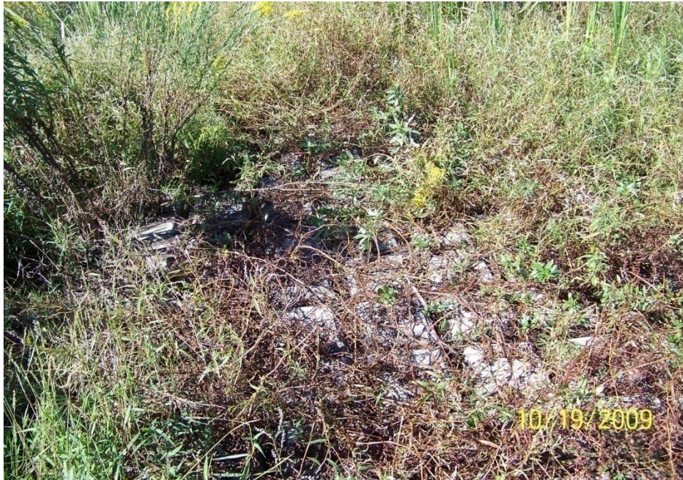
Photo No.23 - Site A2 - armored earthen plug tie-in the bank line on the west end of structure.
