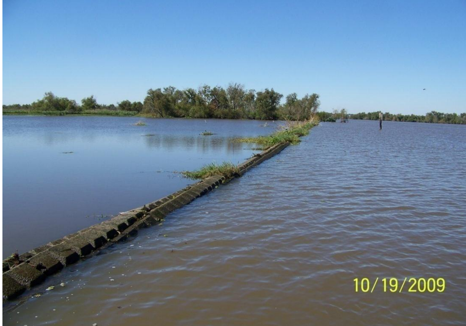
Photo No.53 – Site R1 – view along revetment mats and CPE pipes looking west.
