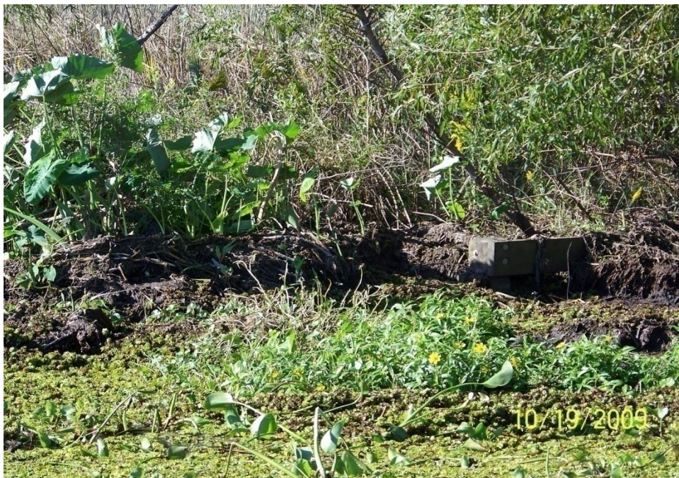
Photo No. 20 – Site F3 – view of heavy vegetation and accretion around timber fence structure.
