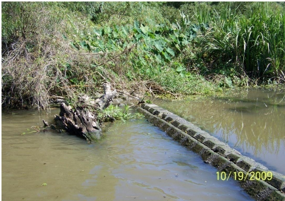
Photo No. 68 – Site R1 – elevated shoreline system tie-in to bank on east side of structure.
