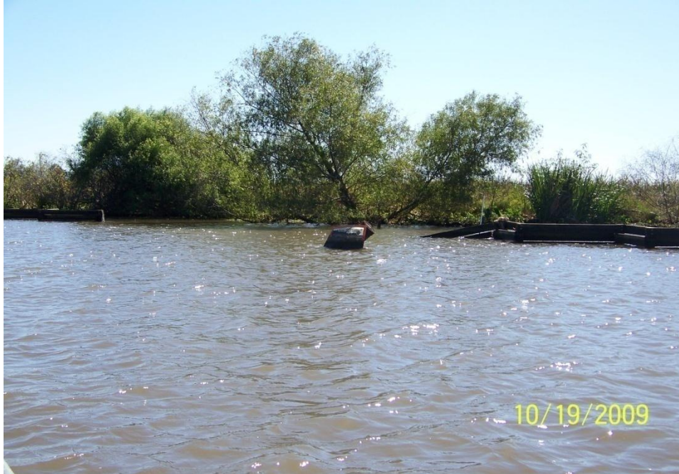
Photo No.33 – Site F2 – view of sign and fence damage by apparent boat collision.
