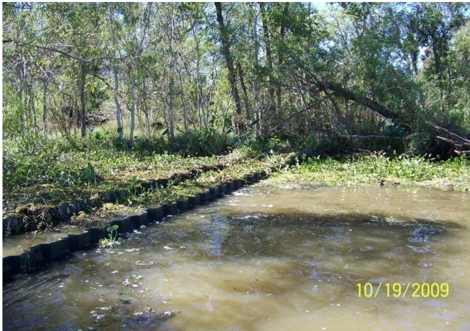
Photo No.60 – Site V1 – fiberglass sheet pile double wall tie-in on the west side of the structure.
