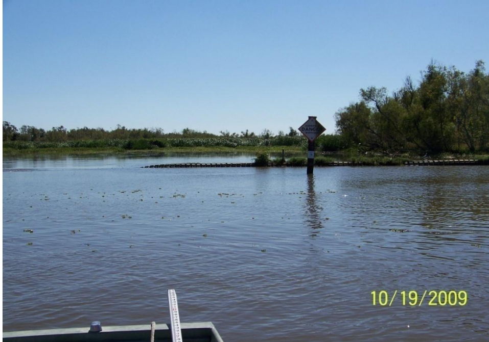
Photo No. 65 – Site R1 – settled area along elevated shoreline system (revetment mats and CPE).
