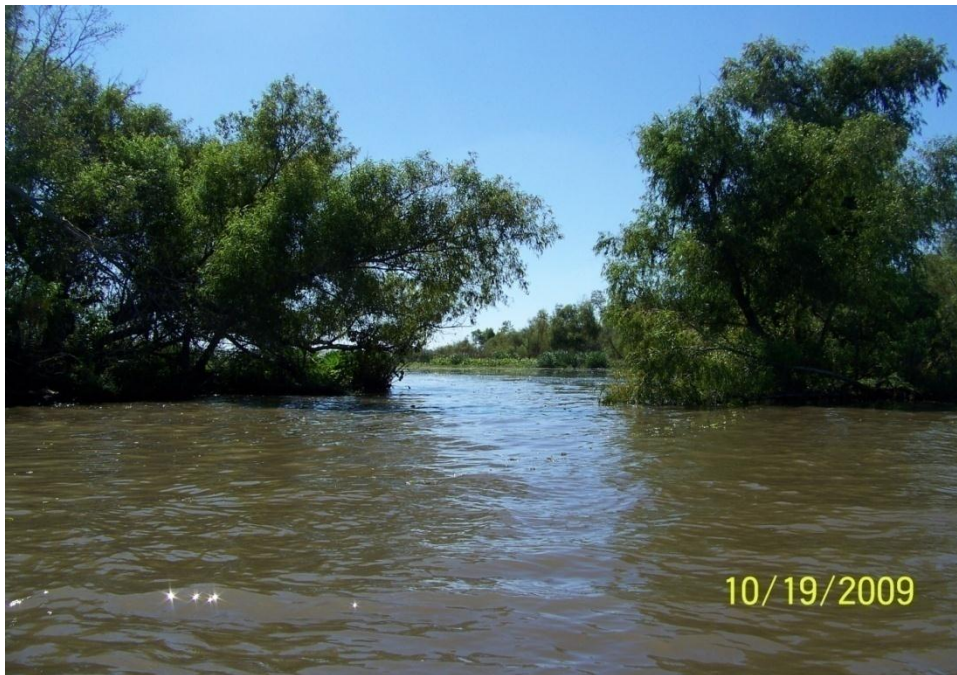
Photo No. 70 – Breach in the bank near the earthen plug east of elevated shoreline unit R1.
