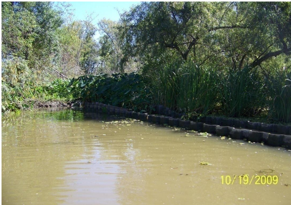
Photo No. 62 – Site V1 – fiberglass sheet pile double wall tie-in on east side of structure.
