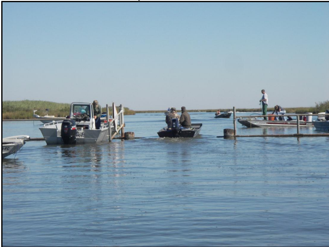
Photo 2, Grand Bayou Weir, close up view showing missing boat guides.
