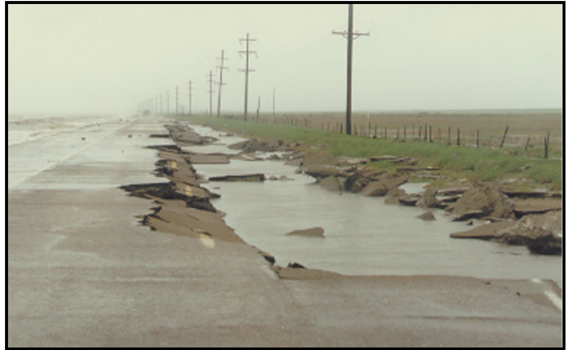
Figure 4. Wave over-wash of the La. Hwy. 82 revetment and roadway during an extreme high tide event showing collapse of the embankment and roadbed beneath the westbound lane of the highway. Image from Underwood et al. (1999).
