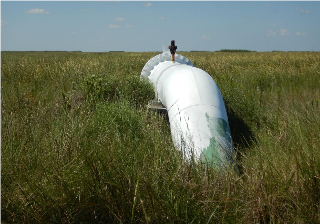
Photo No. 1 , Cycle No. 1, Northeast corner of cell at pipeline riser
