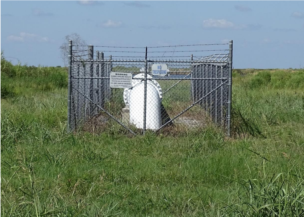
Photo No. 11, West Booster Station – looking West
