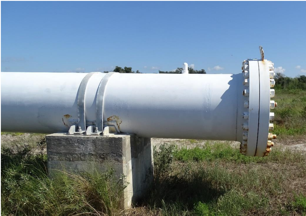
Photo No. 7, East end blind flange/riser, south side of pedestal (looking North)
