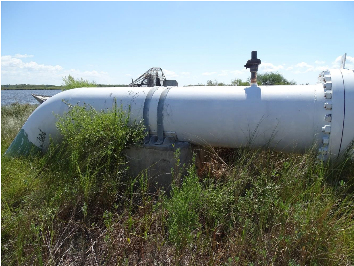
Photo No. 16, South Side of West Blind Flange and Riser looking North
