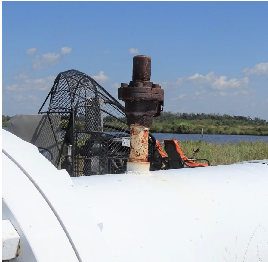
Photo No. 20, West Blind Flange and Riser, Vent Looking South
