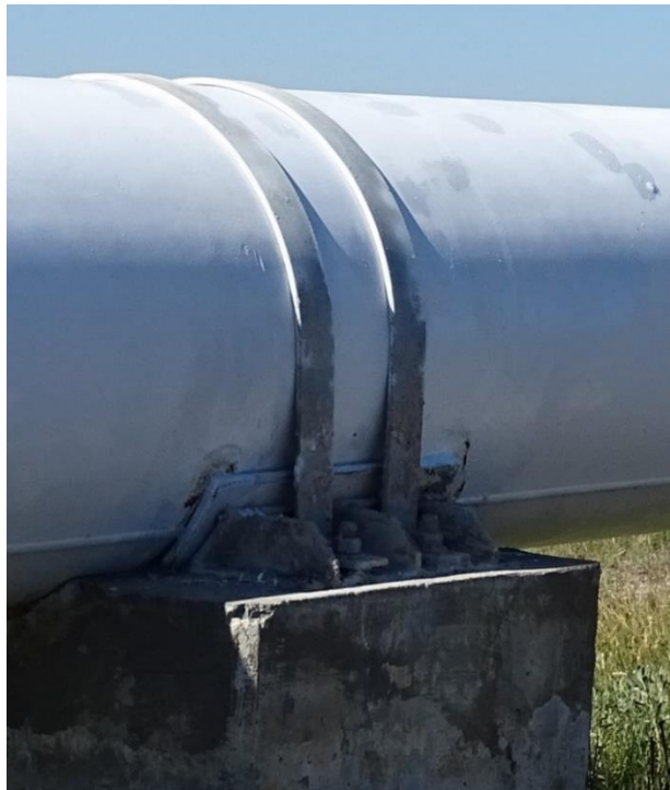
Photo No. 6, East end blind flange and riser, south side of pipeline (looking Northeast)
