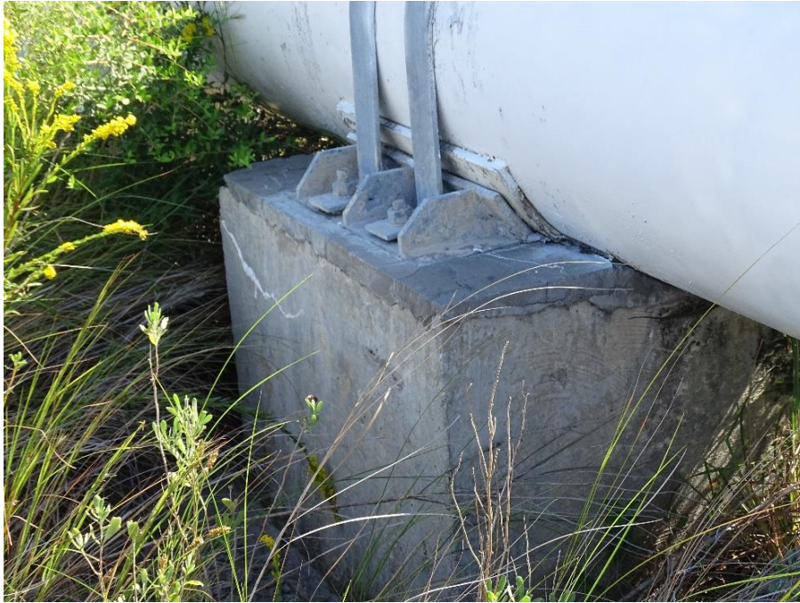
Photo No. 19, West Blind Flange and Riser, South Side – Looking North West (From 2022-2023 Inspection)
