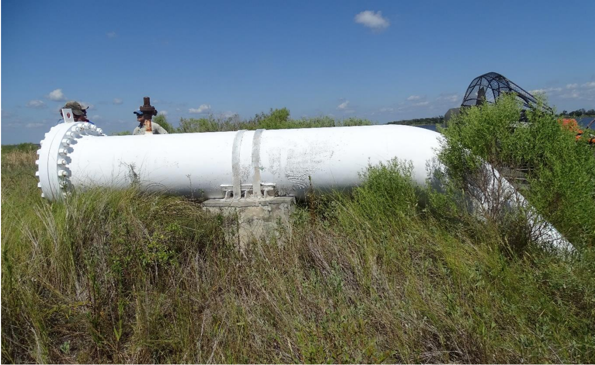
Photo No. 15, North Side of West Blind Flange and Riser looking South
