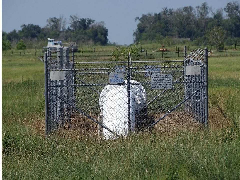
Photo No. 9, East Booster Station – looking west
