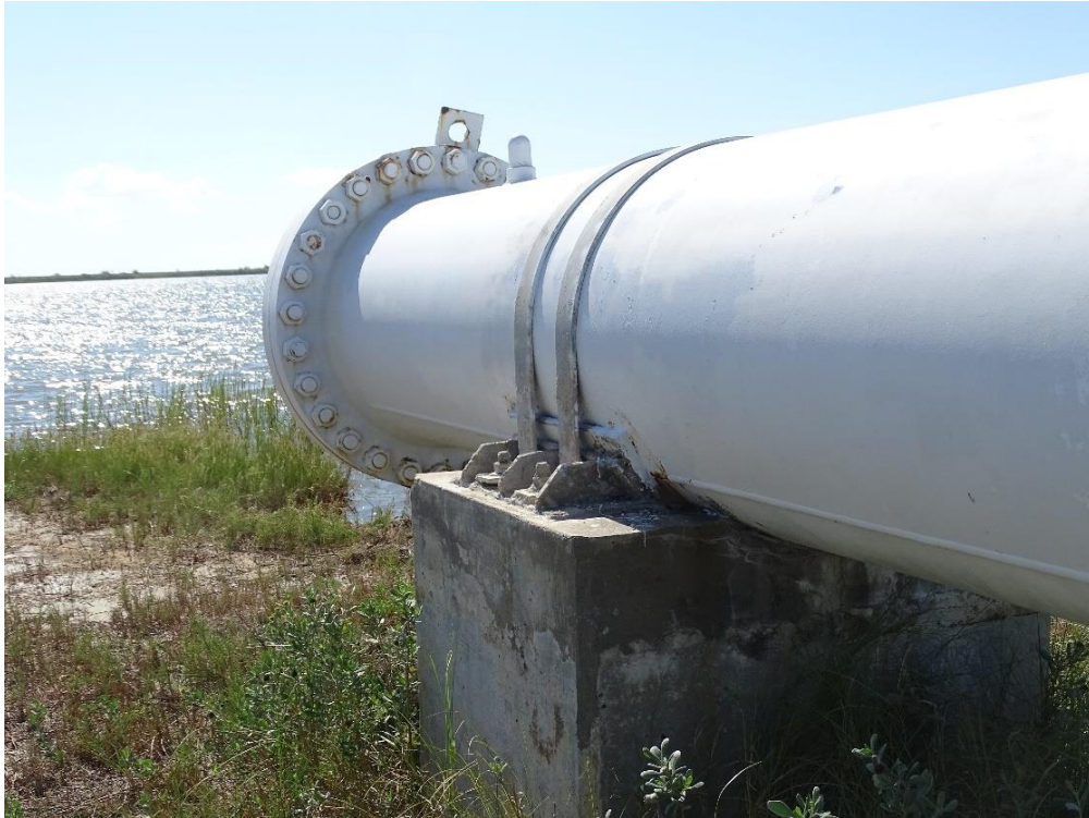
Photo No. 5, East end blind flange and riser, north side of pipeline (looking Southeast)
