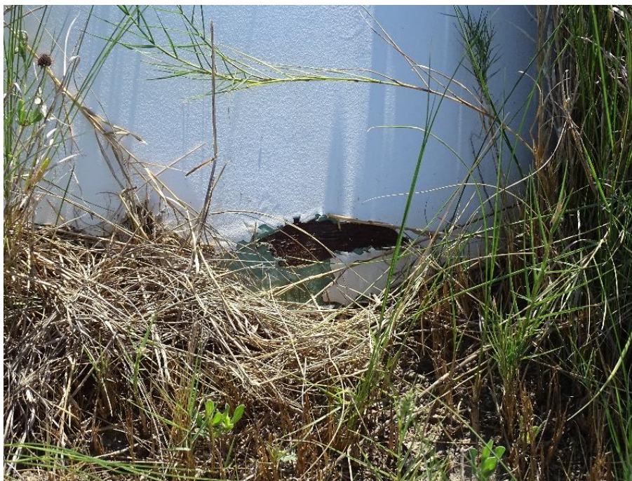
Photo No. 4, Base of East end blind flange and riser (looking East)
