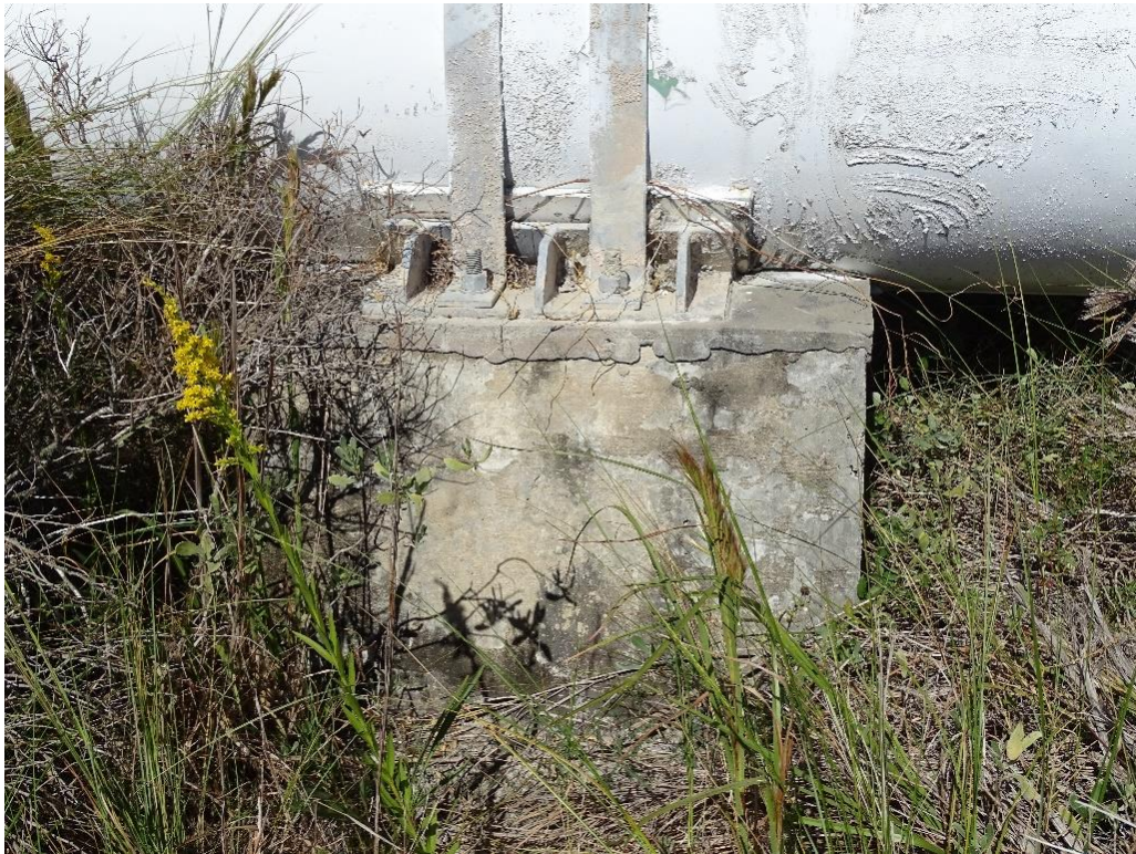
Photo No. 18, West Blind Flange and Riser, North Side – Looking South West (From 2022-2023 Inspection)
