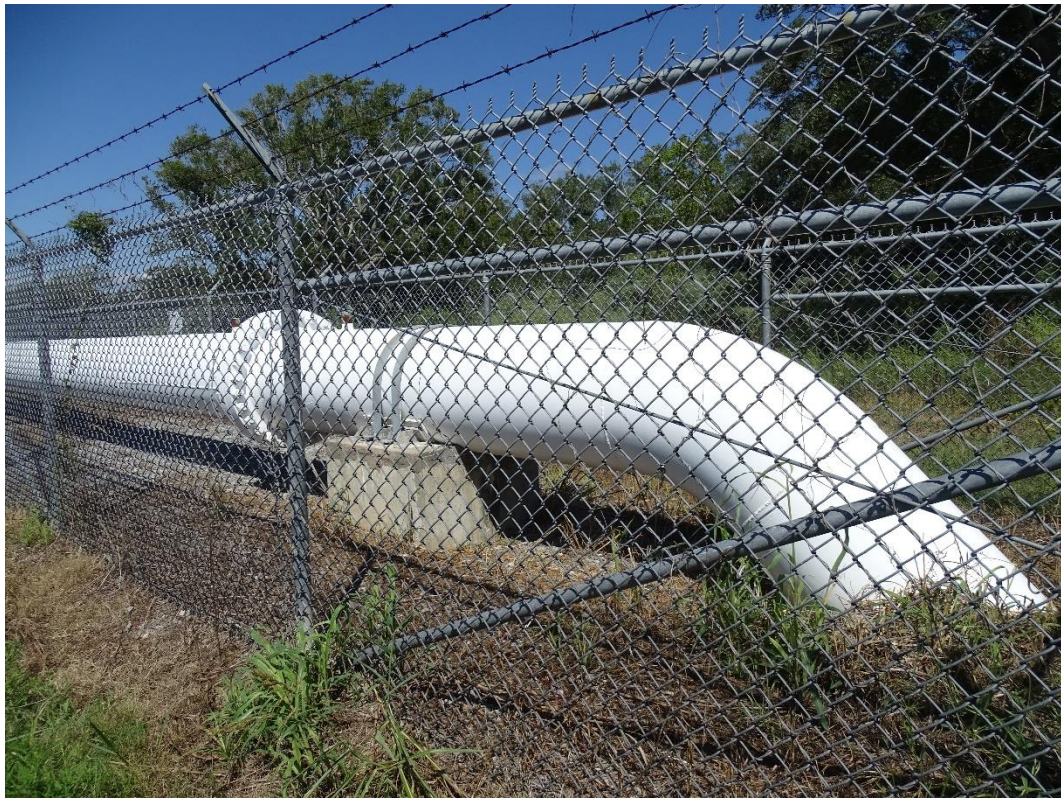
Photo No. 12, West Booster Station – looking Northwest
