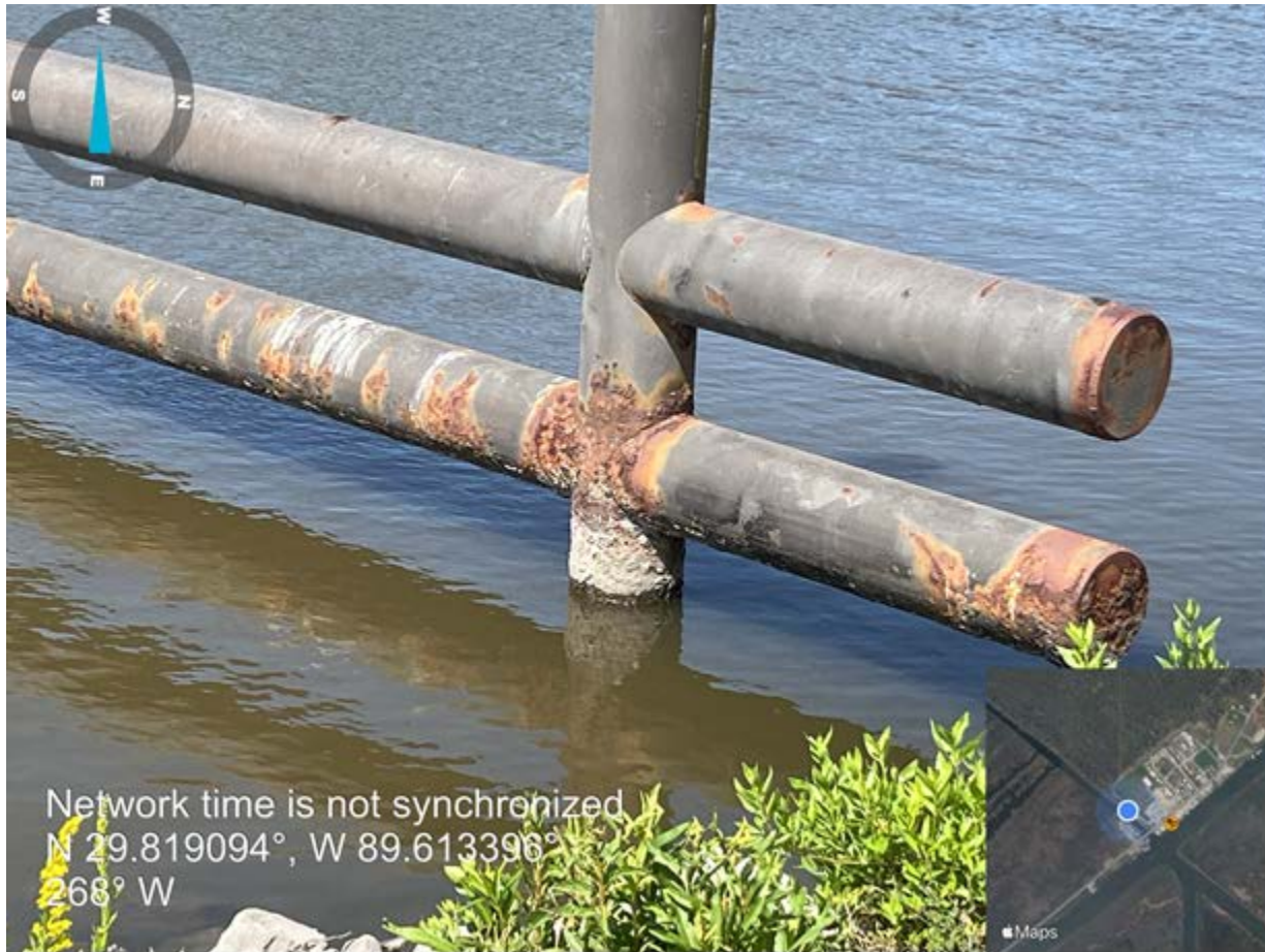
Photo 2. Pipe barrier viewed from project exterior (downstream) on northern bank depicting corrosion.
