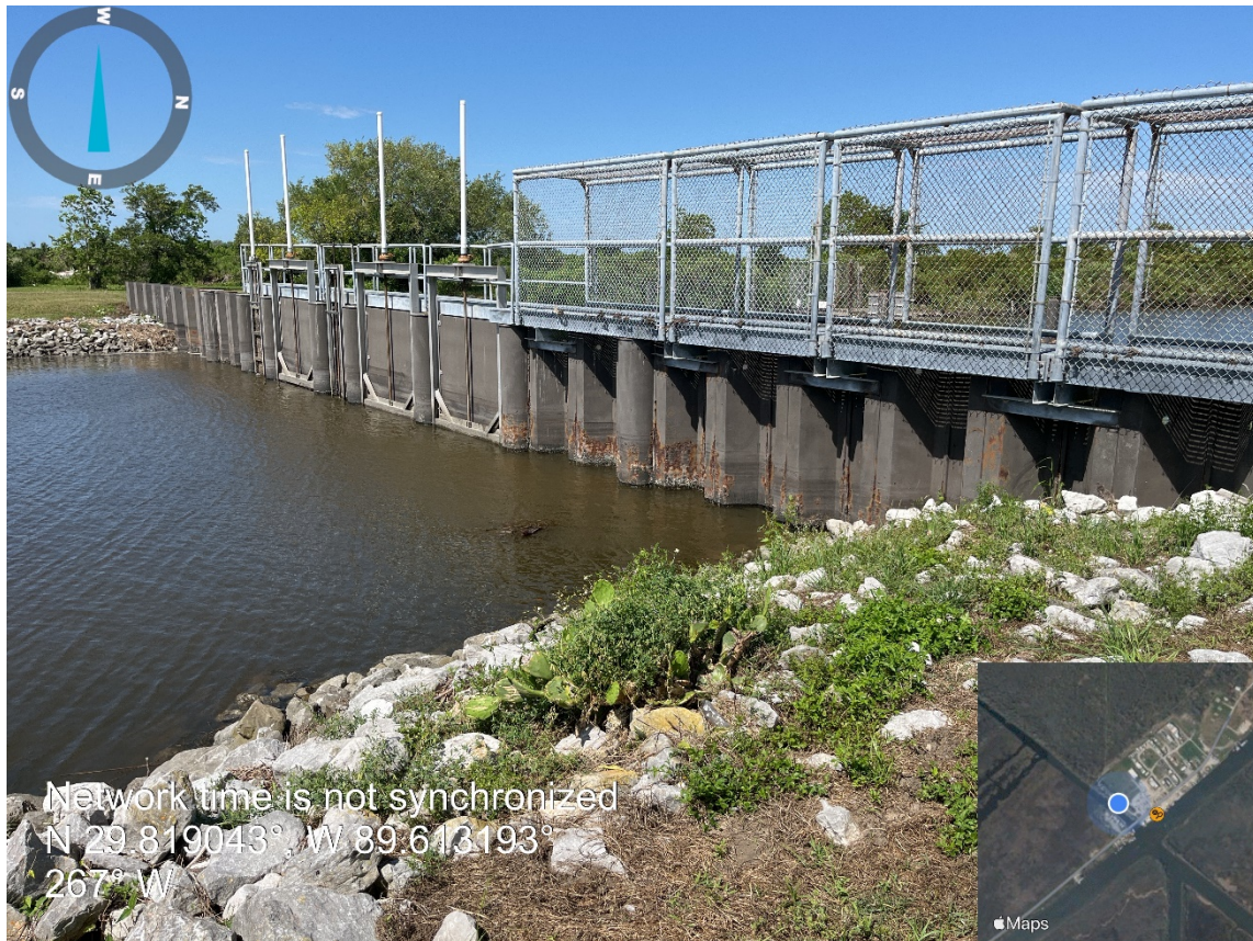
Photo 1. Structure viewed from project exterior (downstream) on northern bank depicting corrosion of the sheet pile structure.
