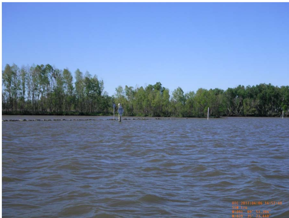
Photo No.12 – view of rock dike and marsh creation site on west side of Bayou Penchant along Bayou Chene near the west tie-in.
