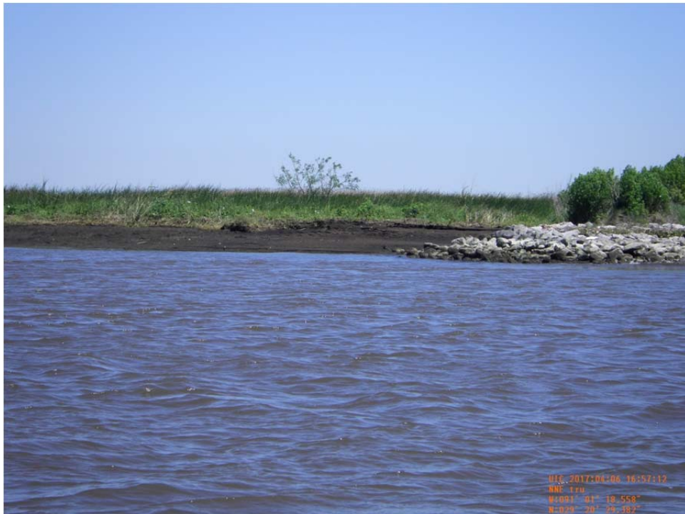
Photo 44- view of rock revetment at the beginning of Reach 1 along west bank of Bayou de Cade at Lost Lake.
