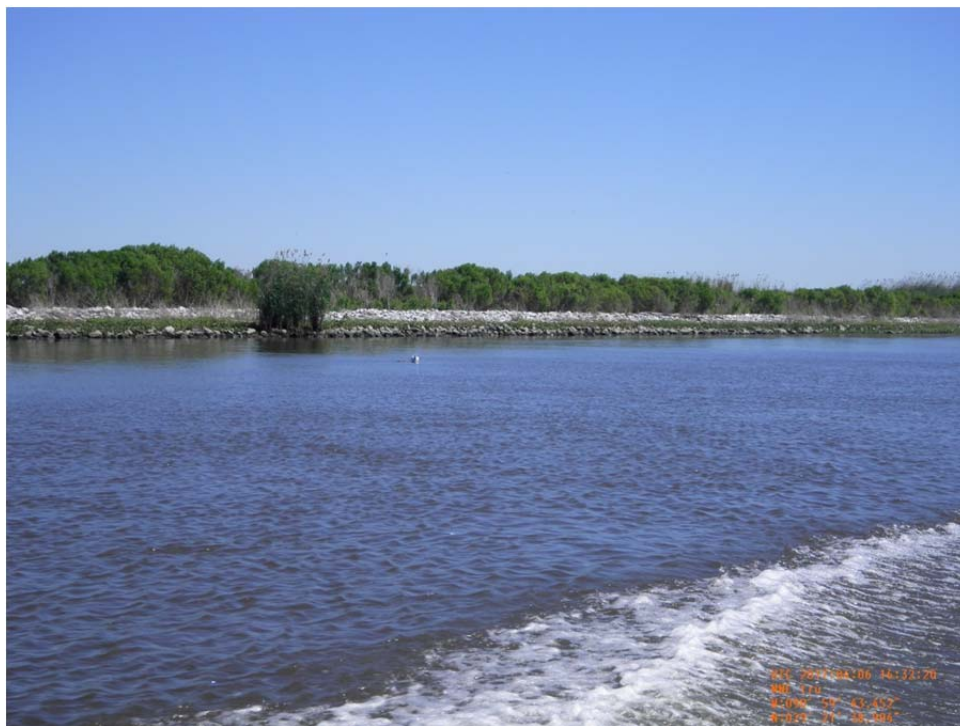
Photo 26- view of rock revetment (Reach 3) along west bank of Bayou de Cade.
