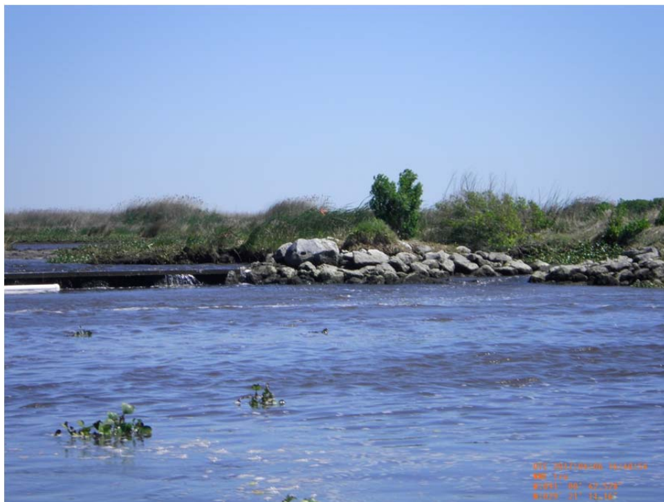
Photo 36- view of north bank tie-in of steel sheetpile Weir No.5 along west bank of Bayou de Cade.
