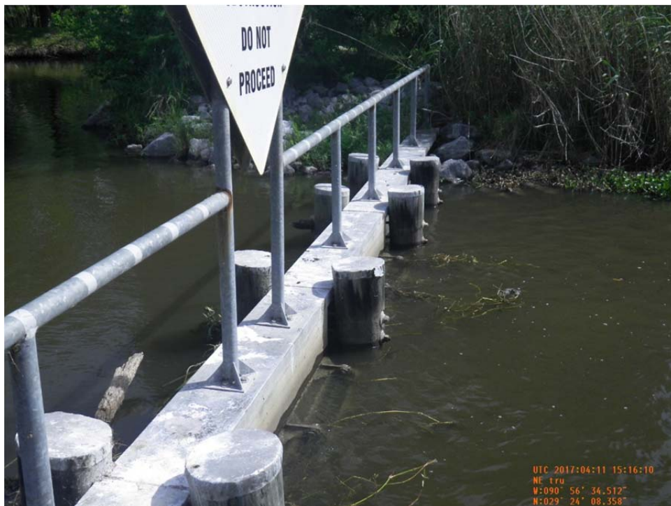
Photo No.24 – view of the channel cap, timber pile supports and sign supports along the Superior Canal Structure.
