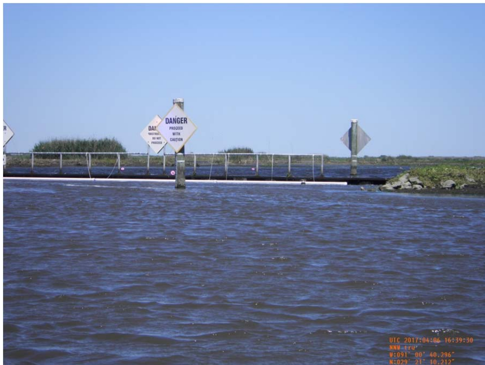
Photo 34- view of steel sheetpile Weir No.5 along west bank of Bayou de Cade.
