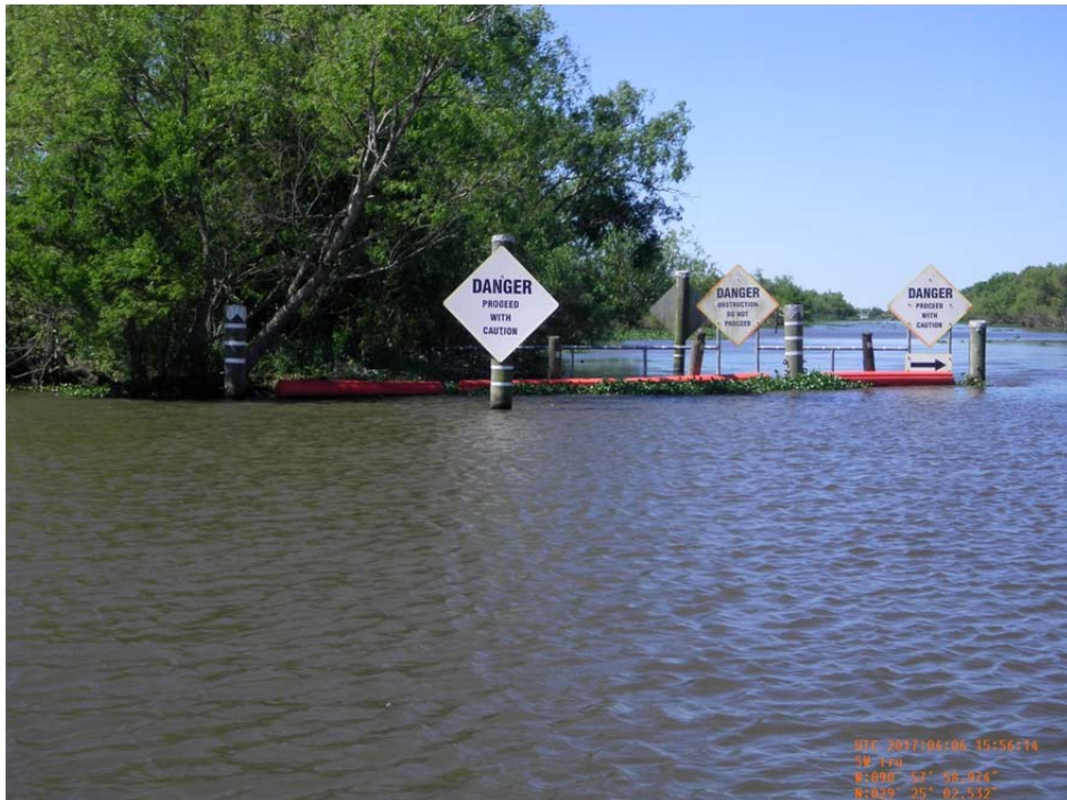
Photo No.14 – view of Brady Canal Structure, debris buoys and warning signs on southeast side of structure.
