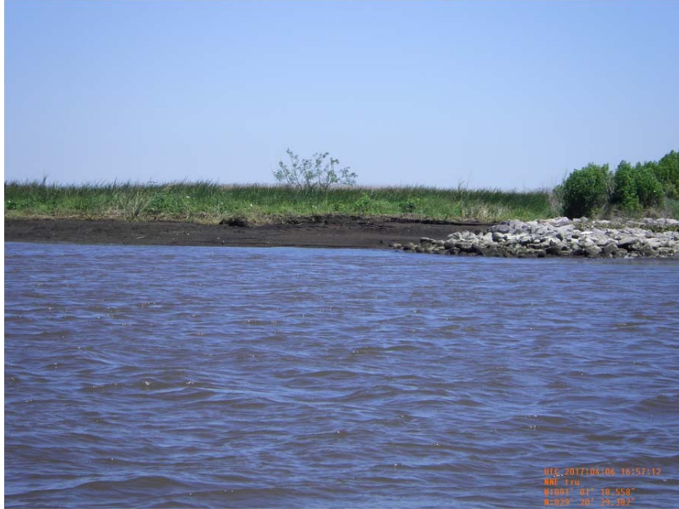
Photo 45- view of rock revetment at the beginning of Reach 1 along west bank of Bayou de Cade at Lost Lake.
