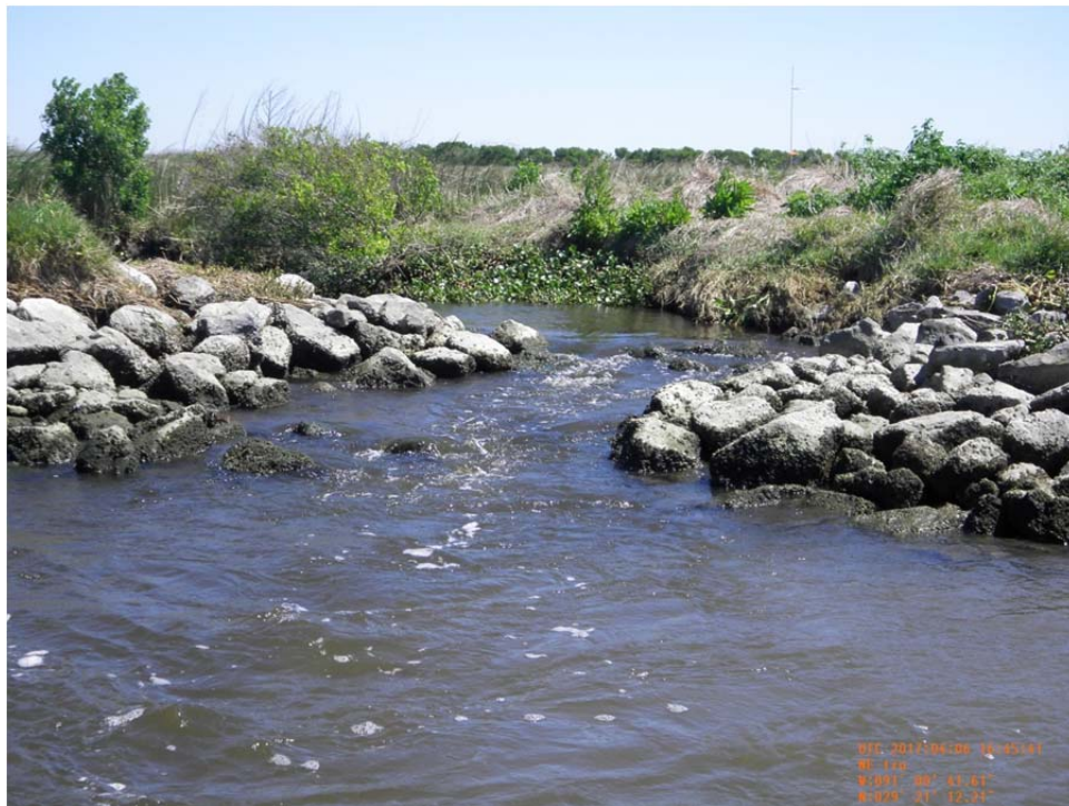
Photo 40- view of cut in rock dike tie-in on the north side steel sheetpile Weir No.5 along west bank of Bayou de Cade.
