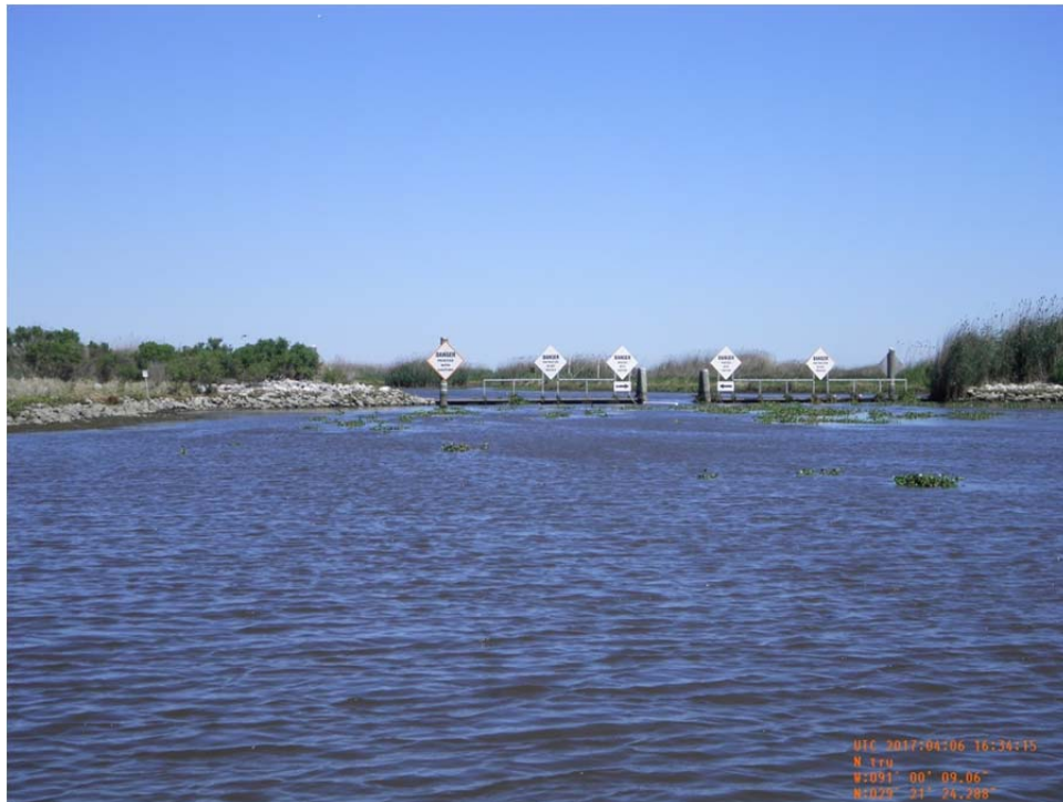
Photo 29- view of steel sheetpile Weir No.4 along west bank of Bayou de Cade.
