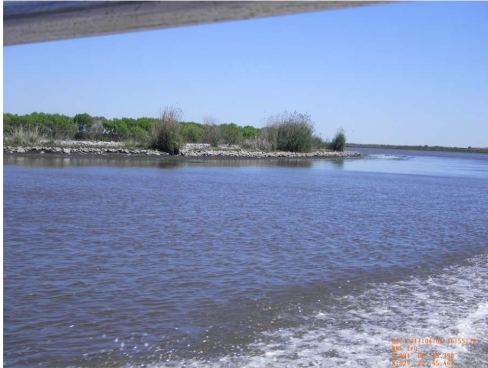
Photo 41- view of rock revetment (Reach 1) along west bank of Bayou de Cade.
