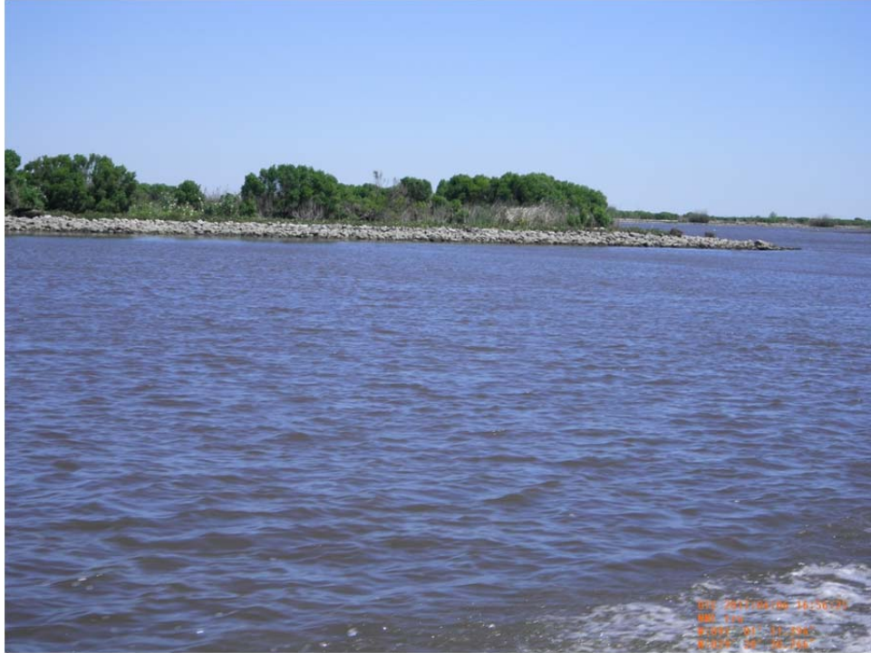
Photo 43- view of rock revetment (Reach 1) along west bank of Bayou de Cade.
