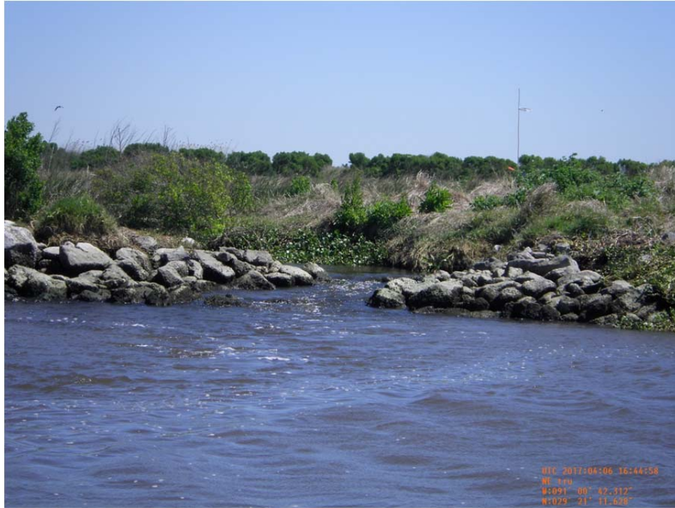
Photo 39- view of cut in rock dike tie-in on the north side steel sheetpile Weir No.5 along west bank of Bayou de Cade.
