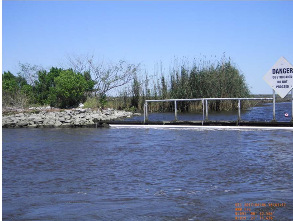
Photo 37- view of south bank tie-in of steel sheetpile Weir No.5 along west bank of Bayou de Cade.
