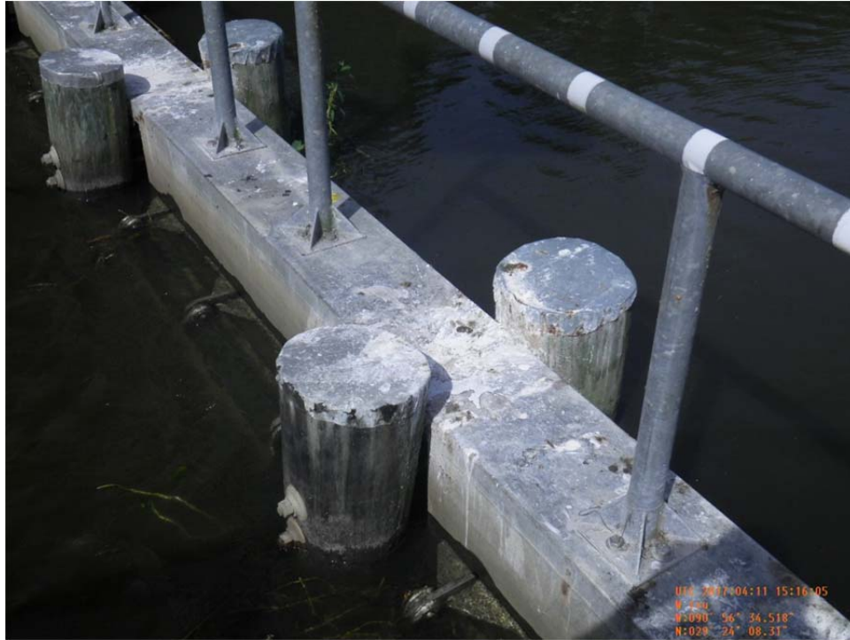
Photo No.23 – view of the channel cap, timber piling and flap-gates on the Superior Canal Structure.
