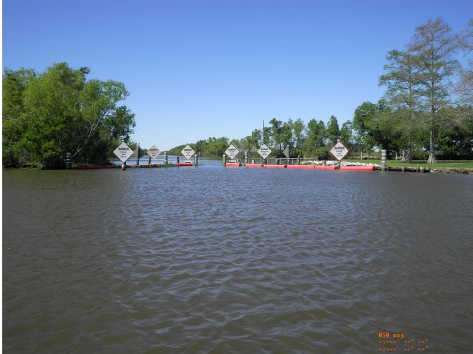
Photo No. 13 – view of Brady Canal Structure at the intersection of Bayou Penchant.
