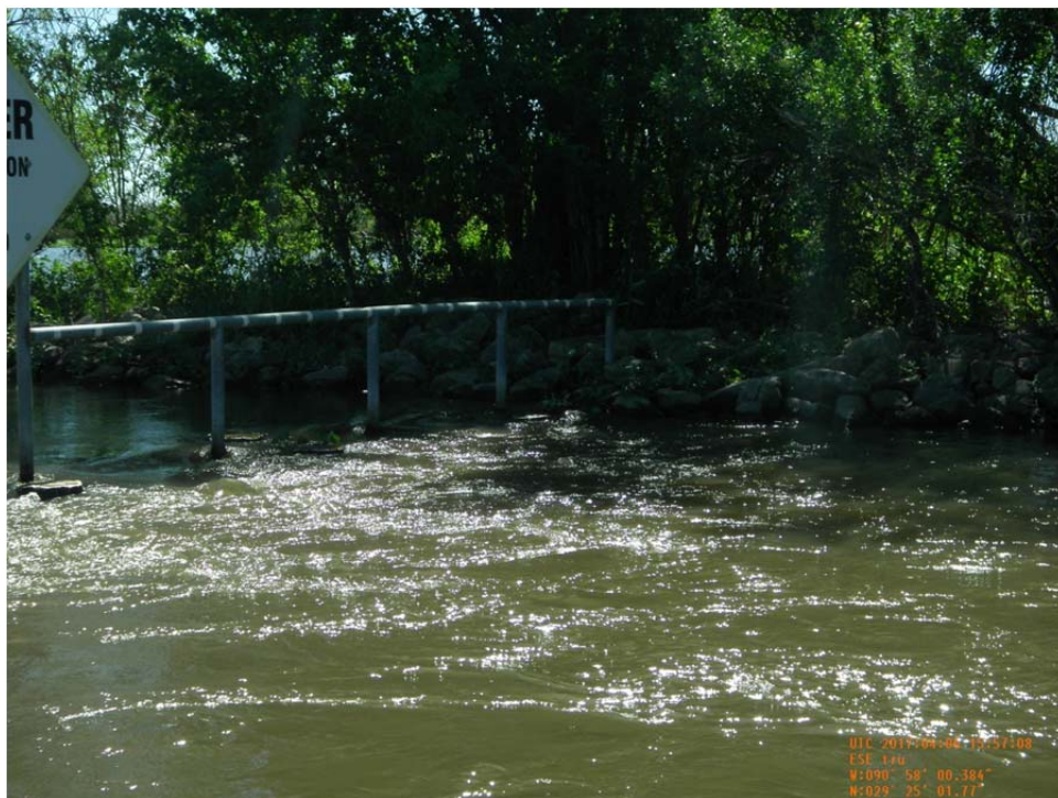
Photo No.16 – view of Brady Canal structure tie-in to the bank on the southeast side of the structure.
