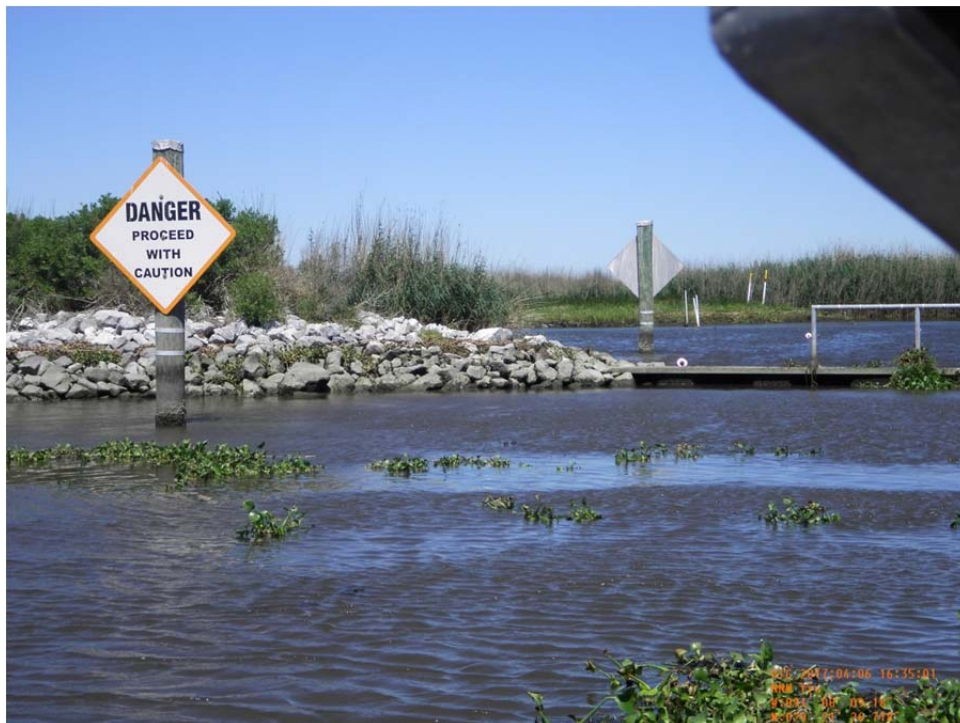
Photo 30- view of south bank tie-in of steel sheetpile Weir No.4 along west bank of Bayou de Cade.
