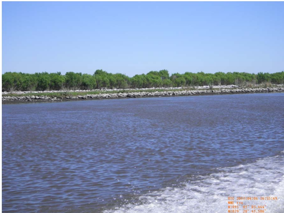
Photo 42- view of rock revetment (Reach 1) along west bank of Bayou de Cade.
