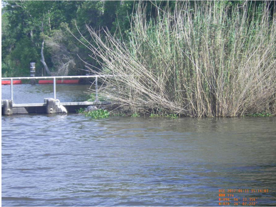
Photo No.19 – view of the Superior Canal Structure and east bank tie-in from the south.
