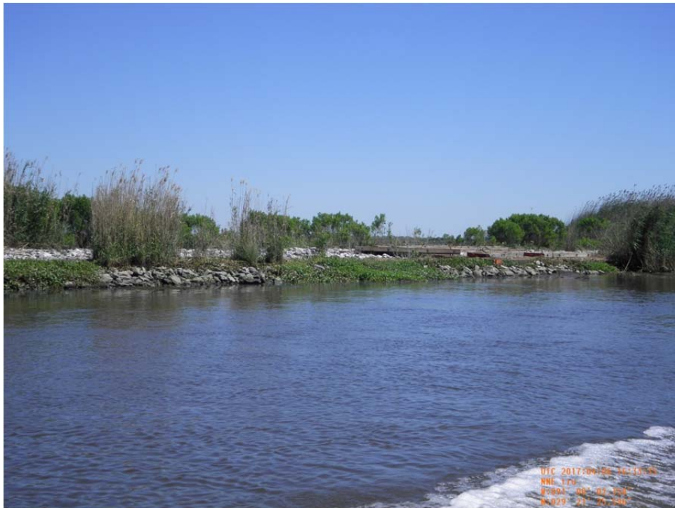
Photo 28- view of rock revetment (Reach 3) along west bank of Bayou de Cade.
