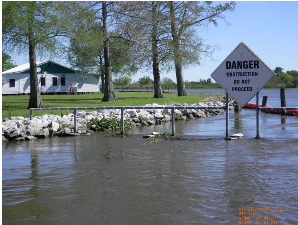
Photo No.17 – view of Brady Canal structure tie-in to the bank on the northwest side of the structure.
