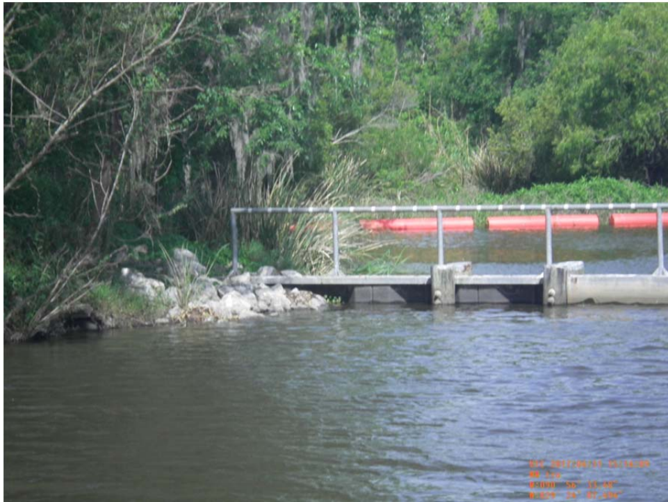
Photo No.20 – view of the Superior Canal Structure and the west bank tie-in from the south.
