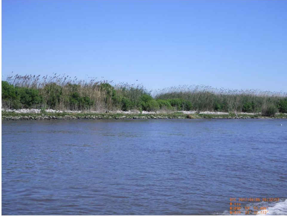
Photo 27- view of rock revetment (Reach 3) along west bank of Bayou de Cade.
