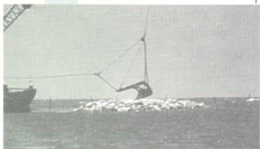
An off-shore breakwater structure is lowered into the water at Raccoon Island.
