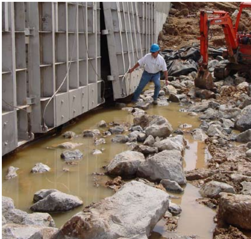
Shown during construction, the gated culverts built under Louisiana Highway 384 restore historic drainage through Black Bayou into Lake Calcasieu. However, the project also provides managers with the option to respond to drought by pinning the gates shut and retaining water in the interior marshes.
